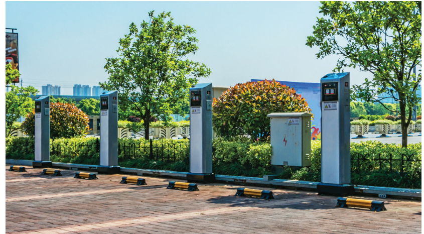
Electric vehicle charging stations.
