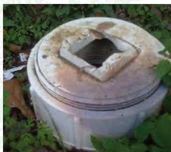
IMPROPERLY CAPPED SEWER CLEANOUT
