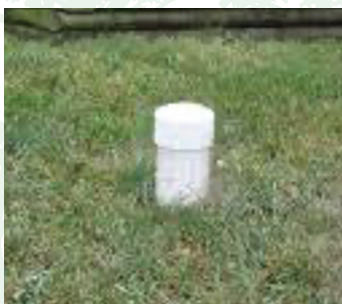
PROPERLY CAPPED SEWER CLEANOUT
